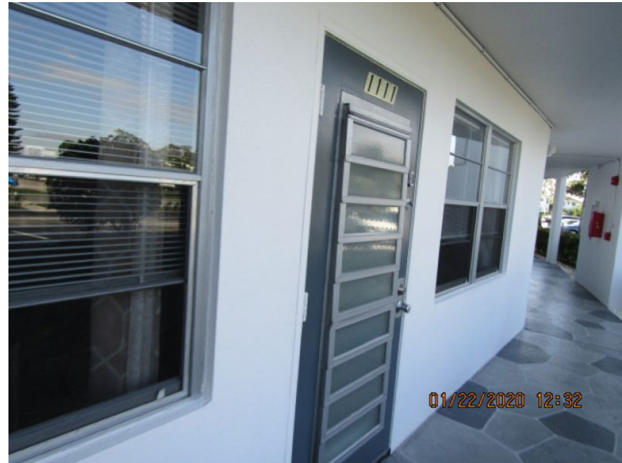
Unprotected Glazed Door
